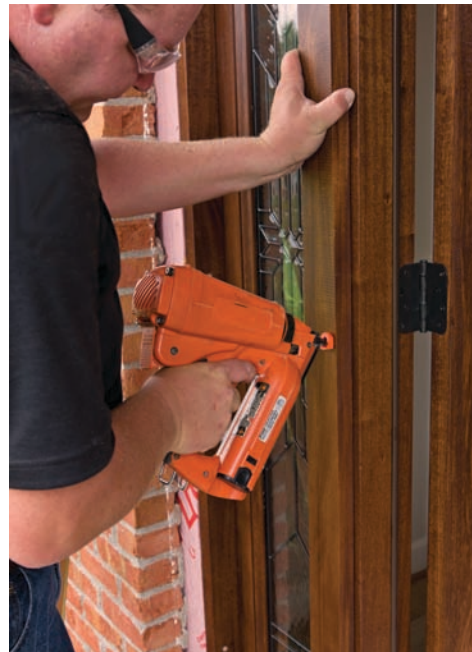
A certified installer employs best practices during installation, ensuring a job well done.
